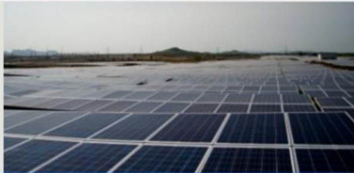
100 MW solar plant in Andhra Pradesh
