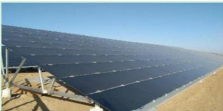
87 MW thin film plant in Bhadla (Fortum)
